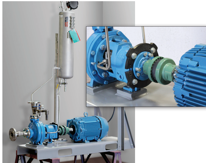
Photos courtesy of GPM Pump and Seal, LLC.
